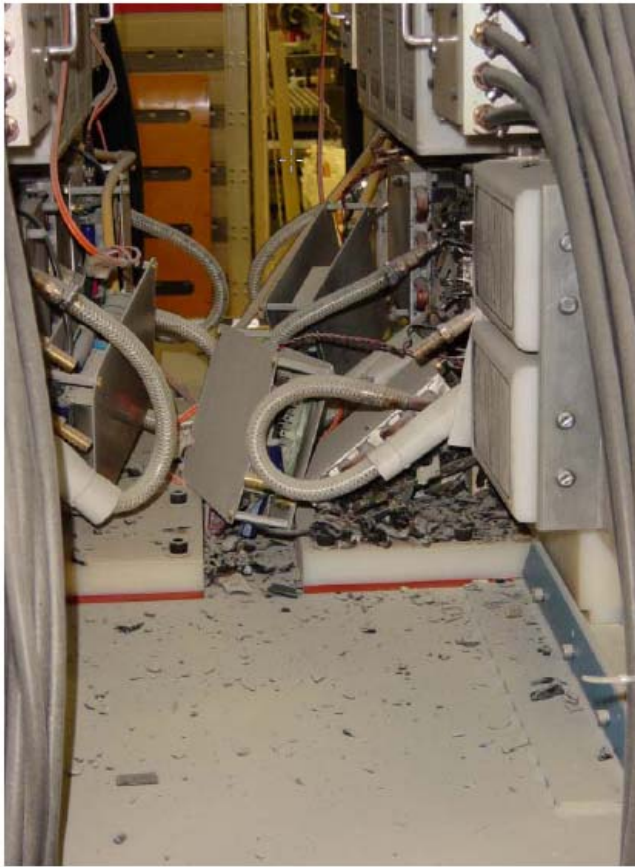
Figure 1: Example of IGBT failure during recent acceptance tests.
